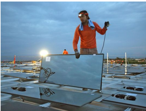
Charlie Quezada installs solar panels at the Palm Springs Air Museum on Sept. 10, 2015. (Photo: Jay Calderon/The Desert Sun)
